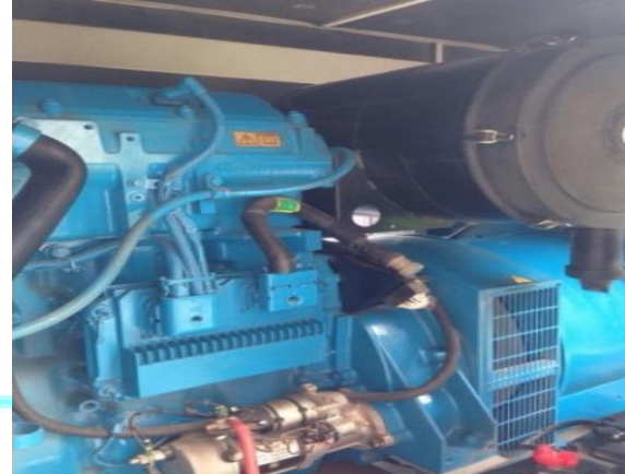
Fig. 3.2: Engine compartment of the power generating plant
