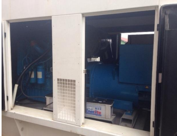
Fig. 3.1: Faculty of Engineering power generating plant
